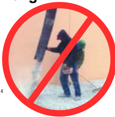
Above: Incorrect positioning especial-
