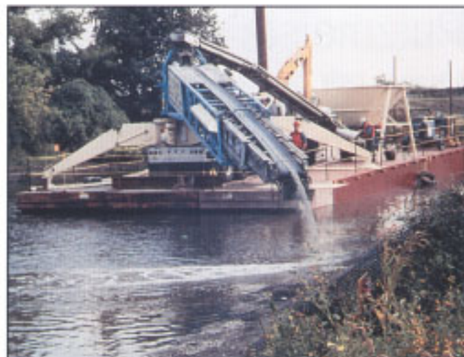
The operator uses radio remote controls to move the belt from side to side to assure even placement of AquaBlok.
