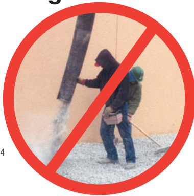
Above: Incorrect positioning especially with the operator at the end hose.
