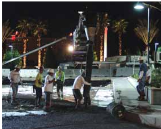
Quinn Concrete Pumping placed pervious concrete for the MGM Residence Towers in Las Vegas for a drive entrance. The pour was easy with their Putzmeister Telebelt® TB 130.
