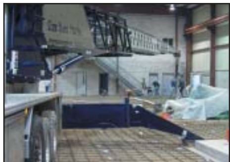
Inside slab - low clearance
