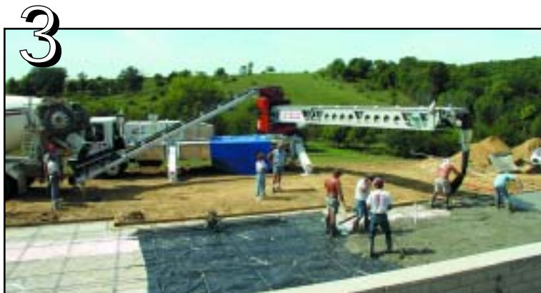
6 Last, the Telebelt places concrete on the slab, and this is still done from the same setup location.
